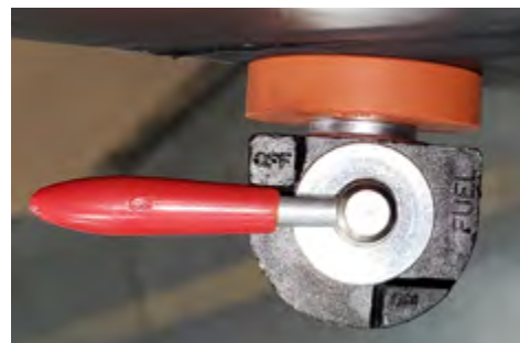
Figure: Fuel Tank Valve, OFF
